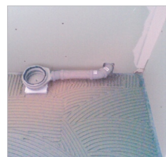
... then the shower base with slope and sealed-in channel is adhered to the substrate element and the drain pot is connected. Joints and transitions are sealed afterwards using sealing tapes from the DRY series.
