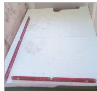
■ Shower during the construction: The substrate element is adhered to the floor with COL-AK fixing adhesive and the recess for the pipework is cut out. The alignment is checked with the spirit level...
