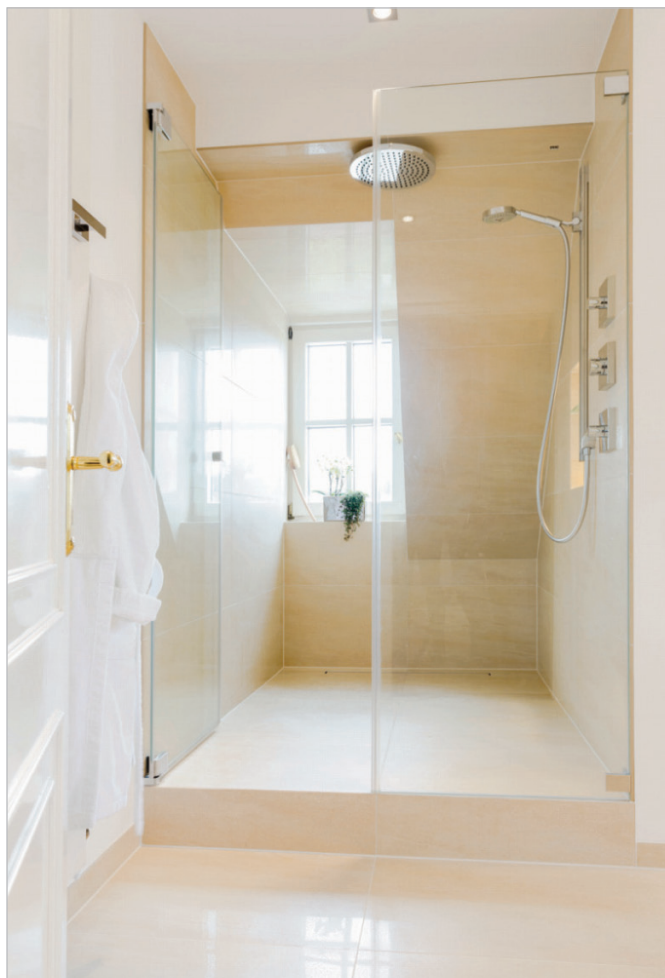
■ Since there was insufficient installation height in the floor for the drain pipework, a step-up solution was chosen.
