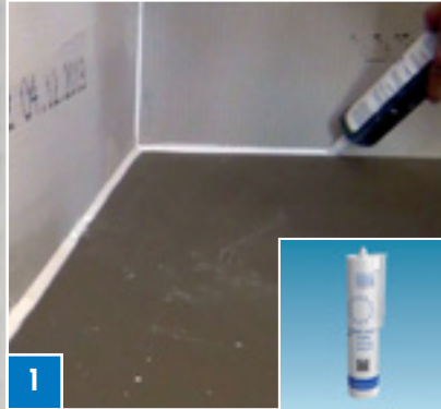
1 Use a continuous strand of COL-MK mounting adhesive to seal the edges of the shower base.
