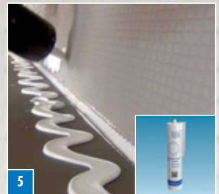
5 Seal the remaining edges of the shower base and the adjacent walls and floors using COL-MK mounting adhesive ...
